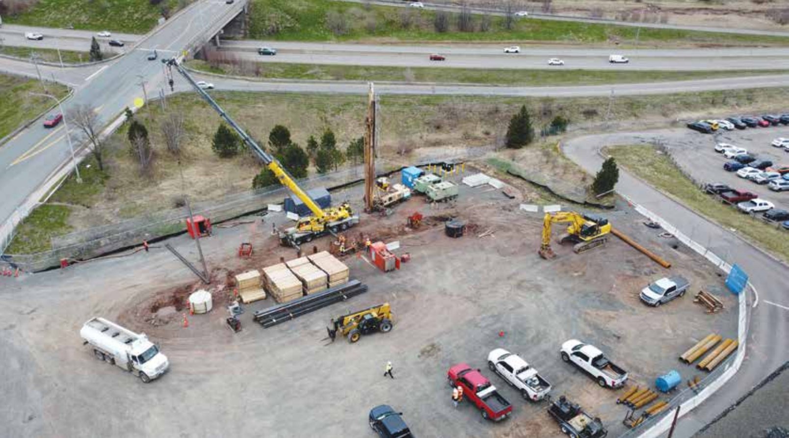
The shoring of the building will be complete sometime in the summer of 2024, after which Phase 1 will begin, which includes the construction of the Science Annex. Completion time for Phase 1 is expected to be about four years.
